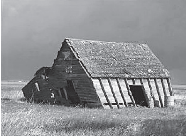
Collapsing barn on former Solomon Doerksen farm. [Bob Derksen]
