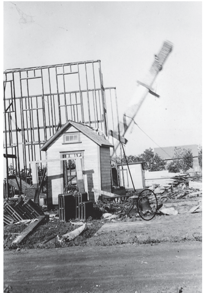
Demolition of the 1912 Rosenfeld school; Circled in black is the school's bell. [Lynne Martel] (See Hedy Mazinke's memoir to find out what happened to the bell.)
